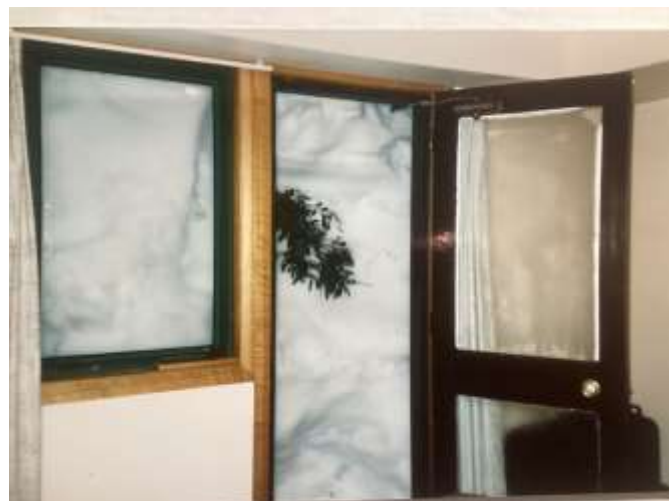
The back door to the games room is completely blocked by snow in this photo. In mid-winter the area between the two wings is filled with snow to the top of the games room roof. The heat of the lodge (even with minimum heat setting when not occupied) melts the snow near the windows & doors and helps prevent them from breaking.
